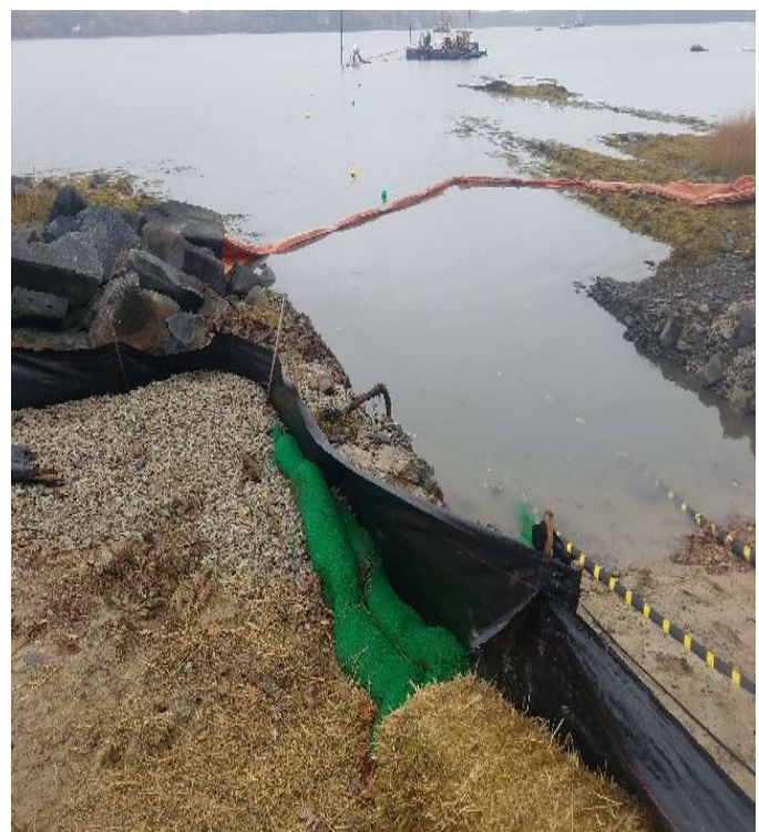
Fig 8: Sediment controls at Getchell property/west side of the Bay. Viewing east. (10-28-19).
