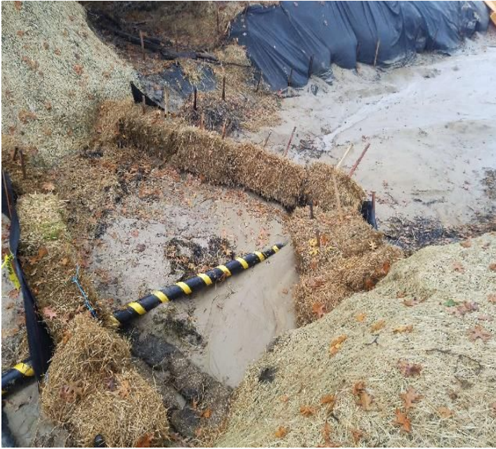
Fig 1: Repairs needed to silt fence and straw bales in trench at Gundalow Landing/east side of the Bay. Viewing south. (10-28-19).
