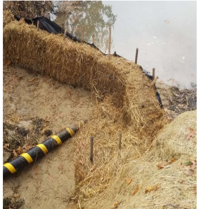
Fig 10: Repairs made to sediment controls in trench at Gundalow Landing/east side of the Bay. Viewing west. (10-28-19).
