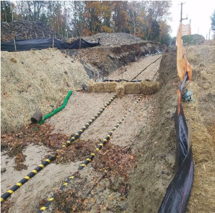
Fig 9: Sediment controls in trench on Getchell property/west side of the Bay. Viewing west. (10-28-19).
