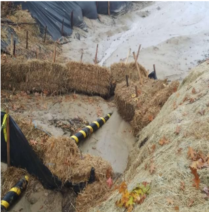
Fig 3: Sediment build up behind silt fence and straw bales at Gundalow Landing/east side of the Bay. Viewing west. (10-28-19).
